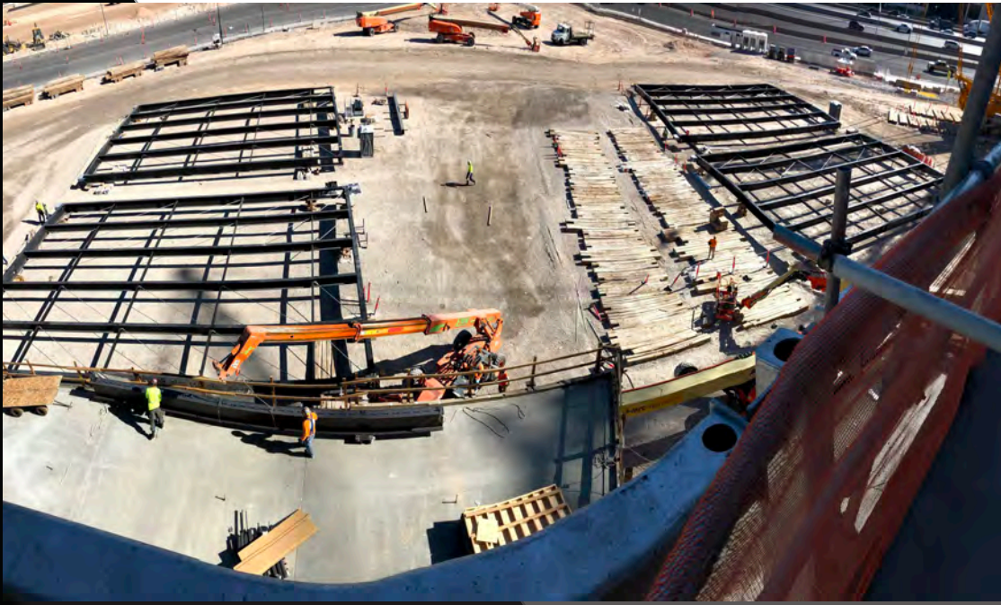
Above: Operable wall panels are being pre-assembled at the north end of the building.
